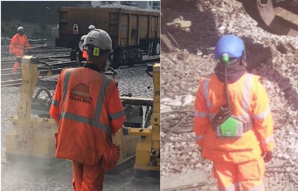
Figure 61 Network Rail photographs showing various types of face mask or ventilator used when handling ballast
